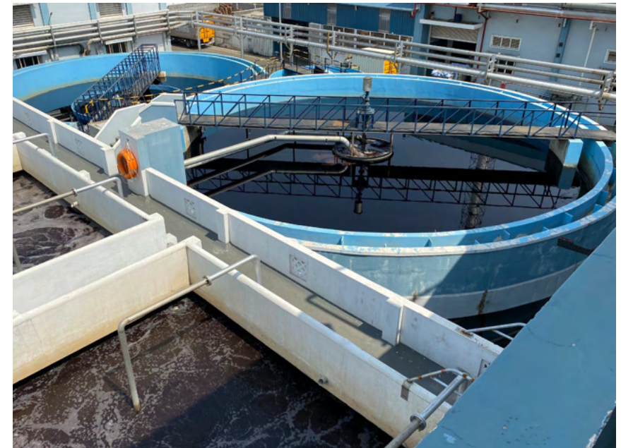
Effluent Treatment Plant in India.
